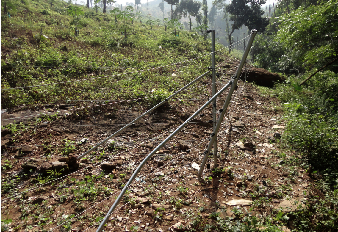
a. Solar electric fence damaged by Asian elephant at Karuvarakundu (Kalikavu Forest Range)
