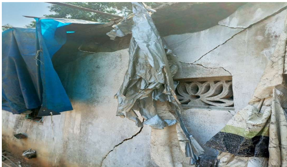
Example of the Poor condition Kavara a house
