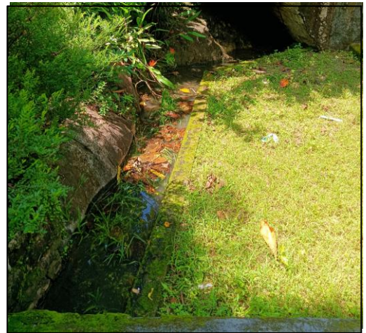
5 (38). Stagnant water in a road-side drainage (Mankayam)
