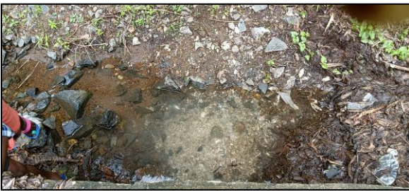
5 (27). Remnant pool in road-side drain (Manjumala)
